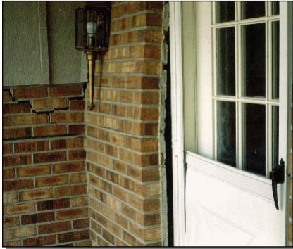
Heave damage, London
