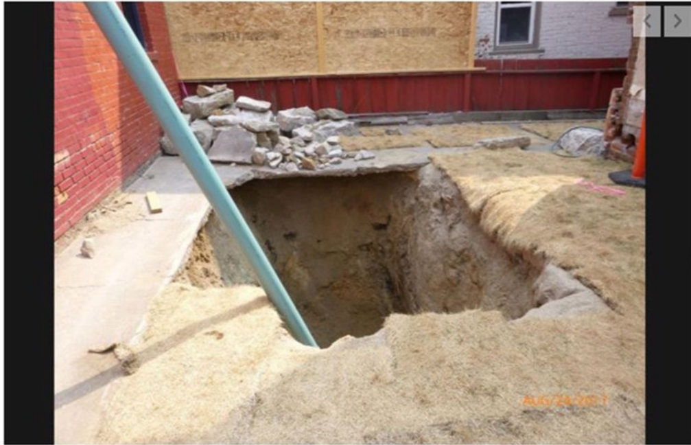
A bedroom was over this spot before the hole opened up on a June night. The homeowners had just had the bedroom torn down a couple of months before.
