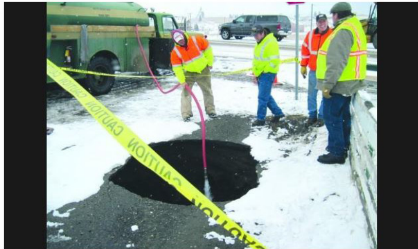
Bob Chansler fills a sink hole with water on a street on Butte's North Side while fellow Butte-Silver Bow road department workers, from left, Tom Loggins and Jim Petritz, and county reclamation director Tom Malloy look on Friday. The hole occurred that morning after an abandoned mineshaft collapsed on 16th Street near Walkerville Avenue. Crews filled the hole with water to see if it would collapse further, and then filled it with concrete and soil.
