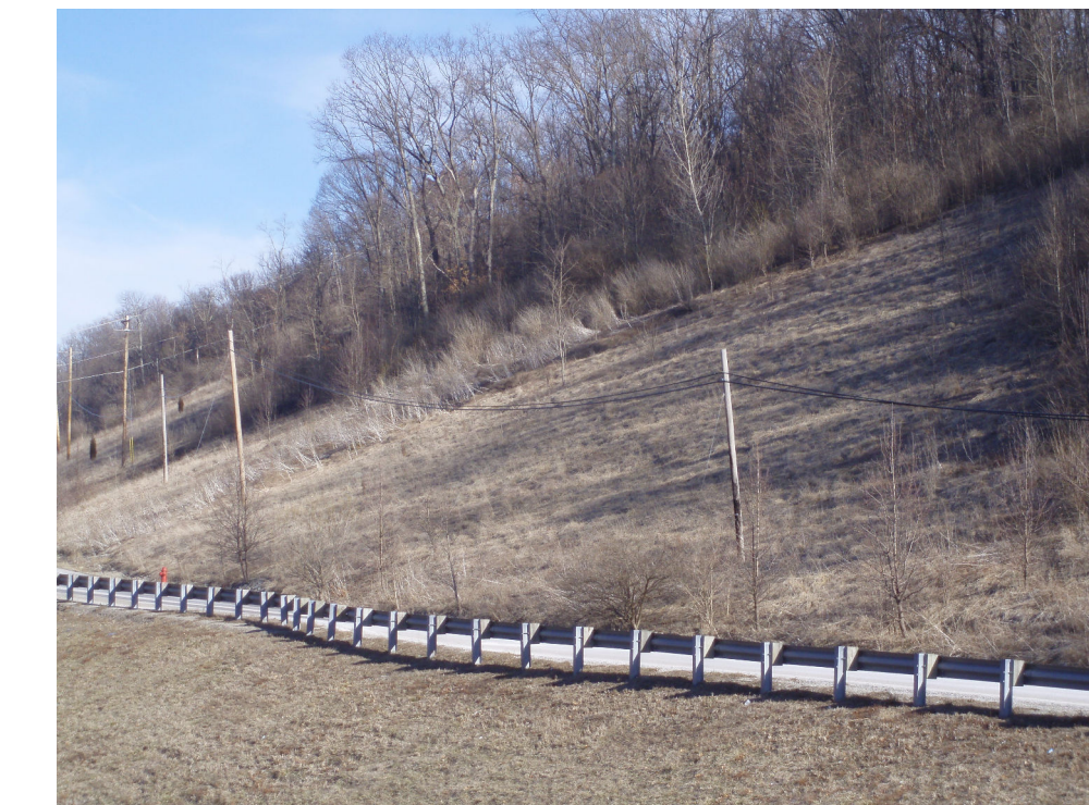
KY 1072: Old embankment failure
