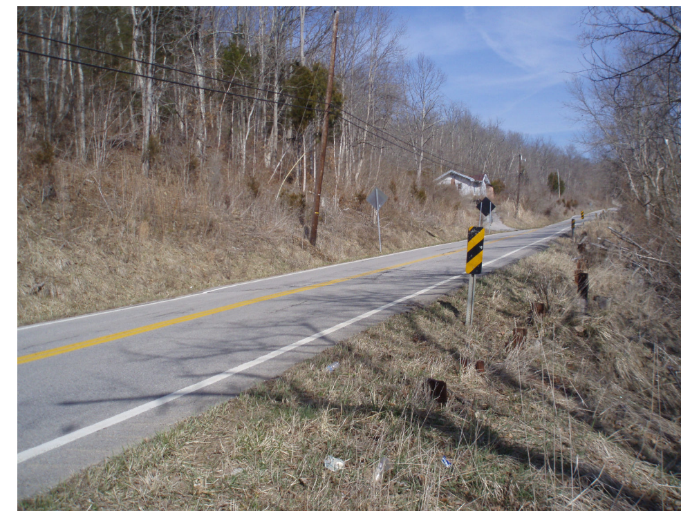
KY 177: Slide above and below road, note old retaining wall.
