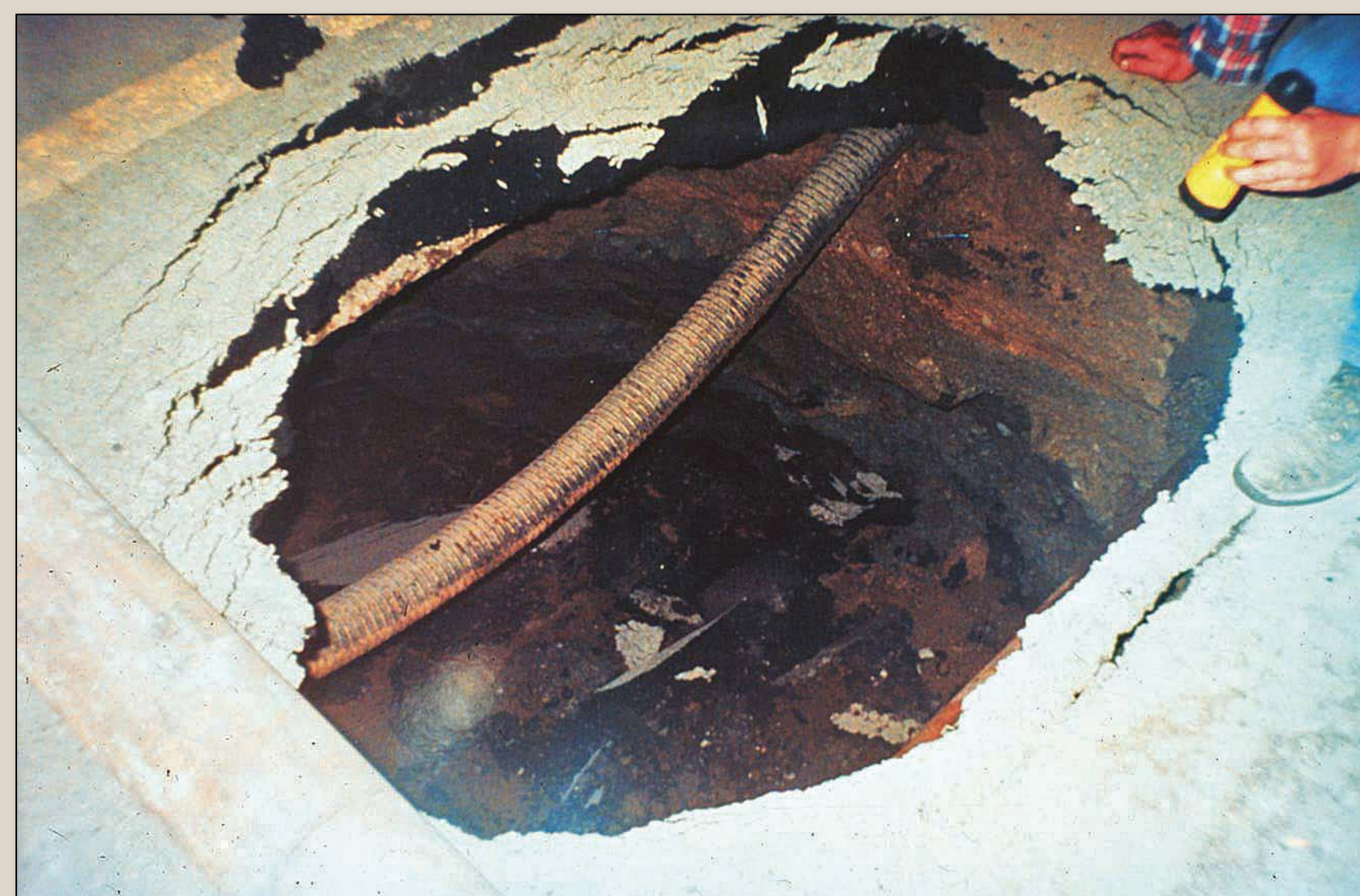
FIGURE 3.—Collapse of Interstate 70, near Cambridge, Ohio, caused by mine subsidence (Crowell, 1995).
