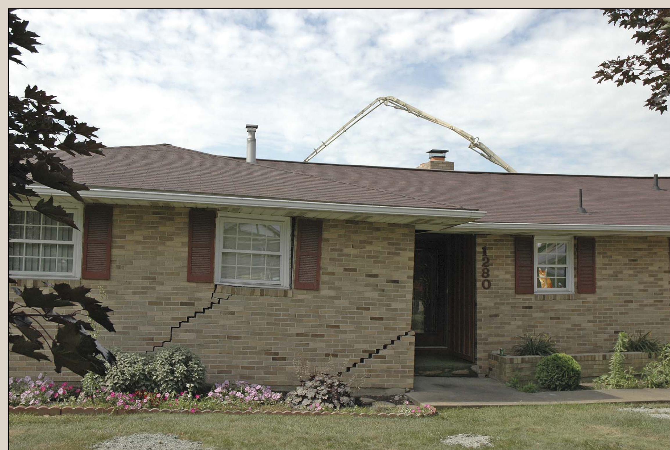
FIGURE 4.—A house damaged by mine subsidence. Sugarcreek Township, Tuscarawas County, Ohio.
